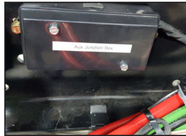
Chassis Electrical Auxiliary Connection
